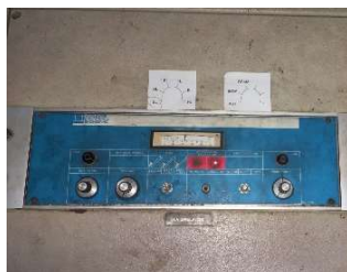
Gambar 4.8 Panel kontrol beban
