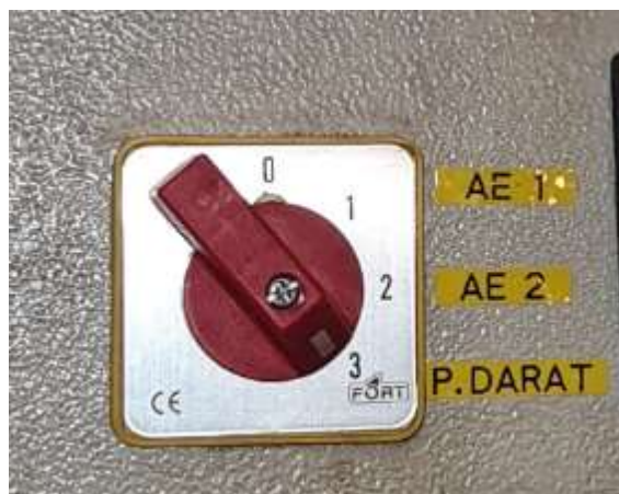
Gambar 3. 4 Selector Swith Generator AE 1, AE 2 dan Power Darat
