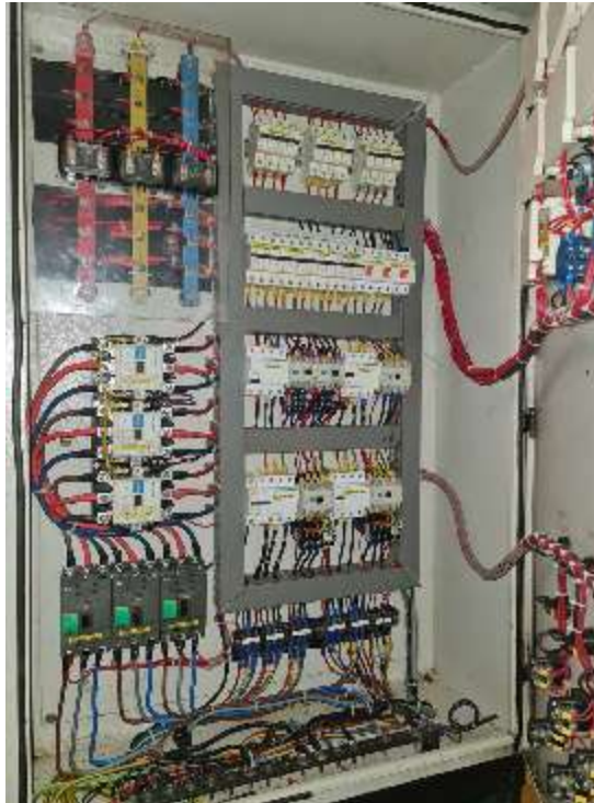
Gambar 3. 3 Panel listrik shore connection di kapal MRP 19
