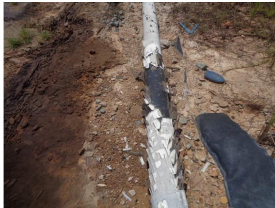
Gambar 1.1 wrapping rusak pipa underground NKL-1061
